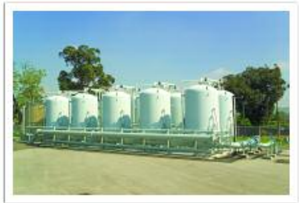
GAC vessels at Central Basin's Water Quality Protection Project.
