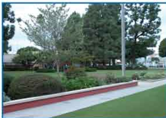
Landscape irrigation controllers installed at the City of Gardena's City Hall
