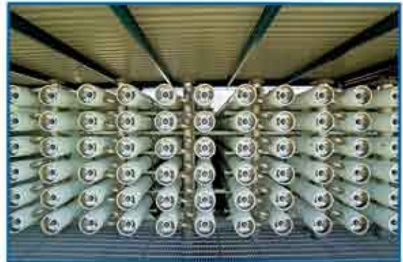
Reverse Osmosis Units
