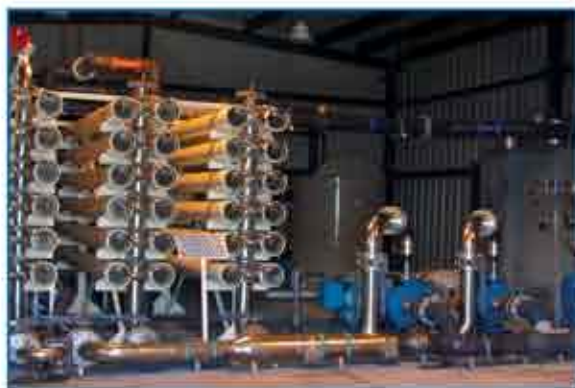
Brewer Desalter RO treatment onsite
