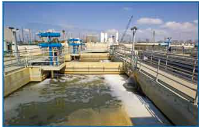
Recycled water filters at West Basin's Water Recycling Facility
