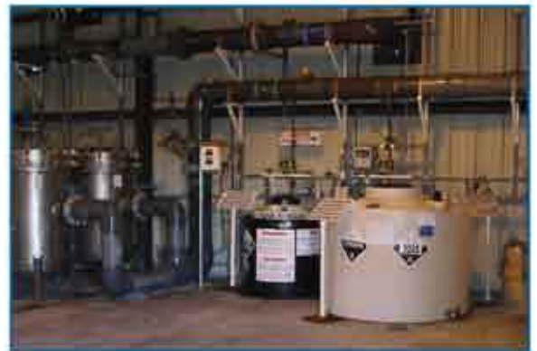
Chemical addition tanks located inside the RO building
