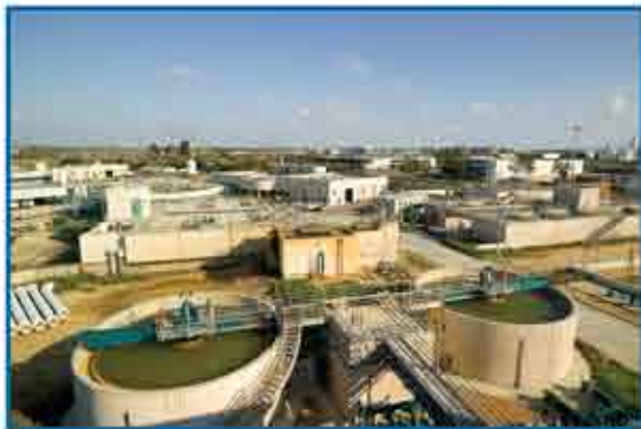
Gravity thickener tanks at the West Basin Water Recycling Facility
